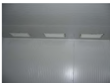
c- Air channels located on the ceiling
