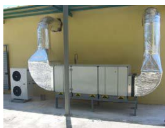
d-Air conditioning unit
