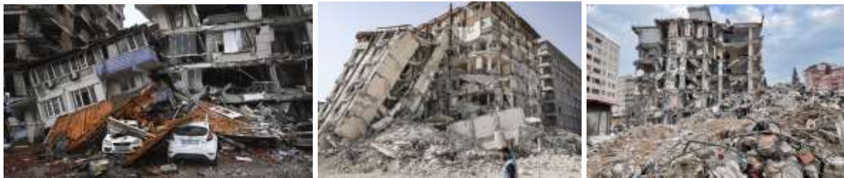
Figure 1. Examples of damages of buildings in the 6th February 2023 Türkiye earthquake (URL1, URL2, URL3)
